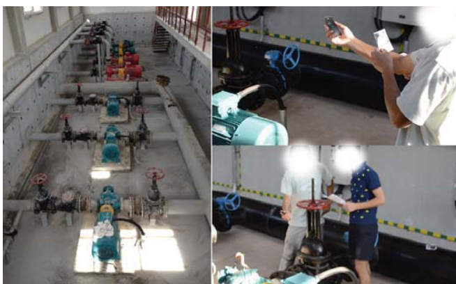
Fig. 5 Integrated pump house and pump test
